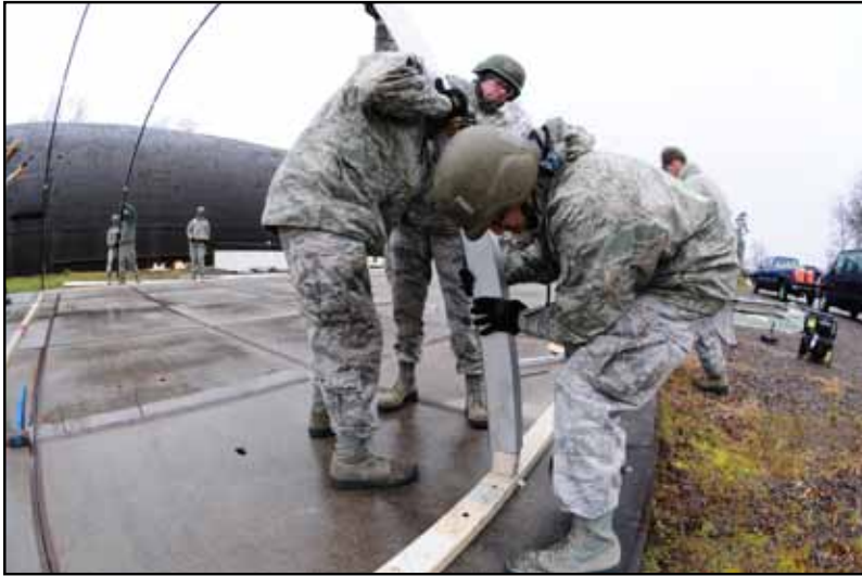
Civil Engineer structural specialists build a large tent at Silver Flag 2016 in Ramstein Air Base, March 8. The large tent is used as a dining facility during the exercise deployment.
